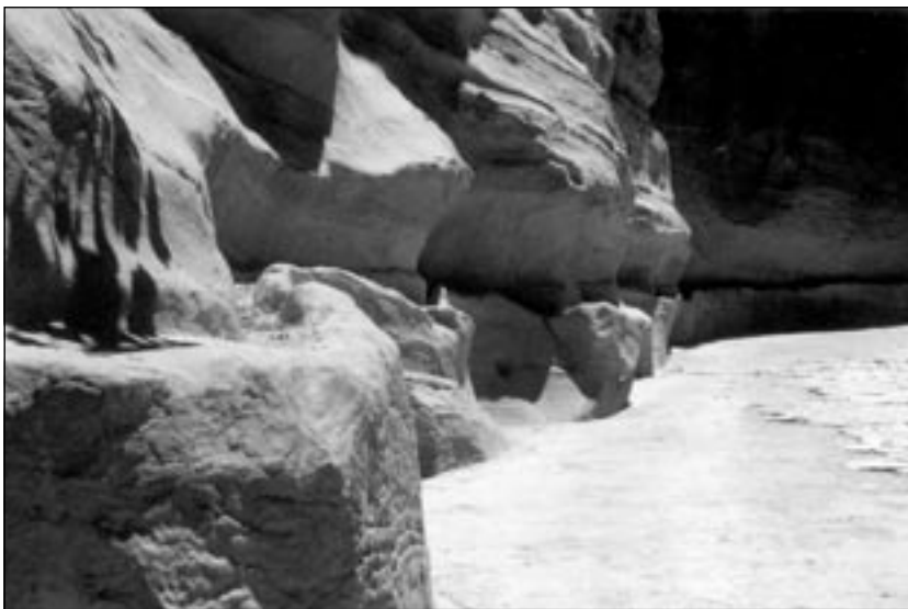
Figure 5b. Channel trough on the north side of the Siq for placement of piping.
